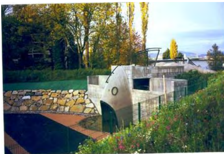
Figure 23 Bassin de stockage-restitution
